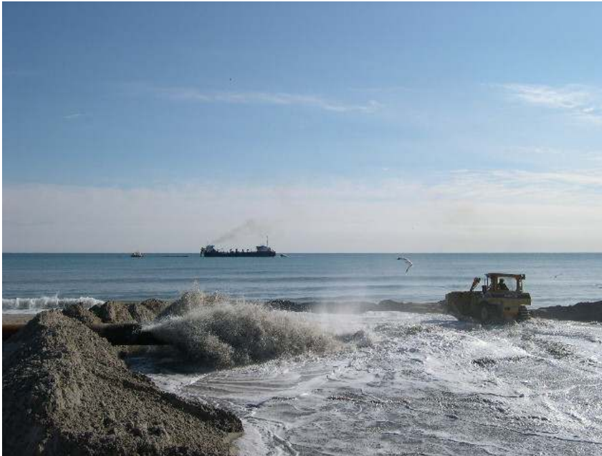
Beach nourishment in action - Pine Knoll Shores, 2007. Sand is pumped to the beach via long pipelines in a water/sand mixture called a slurry – the water drains off the beach while the weight of the sand helps the material stay in place. Bulldozers are subsequently used to contour the sand into the engineered beach design. Note the hopper dredge pumping sand in the background.
